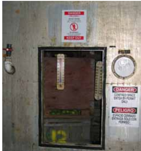
Figure 6. All doors to the CA rooms in the facility have the required Confined Space signs (in Spanish and English) affixed
