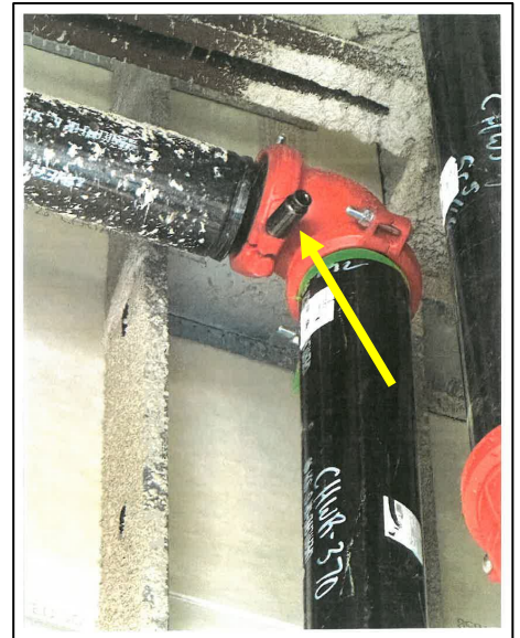
View of grooved pipe end separated to insert end cap into elbow to isolate for pressure testing. The socket remained on the coupling bolt being loosened (yellow arrow). The end cap ejected under 150 psi compressed air pressure. Case 23MI139
