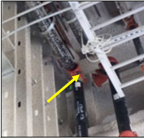
View of elbow (red) where end cap dislodged under pressure. Case 23MI139.
