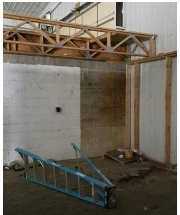
Photo from MIFACE report 18MI105 . The duty rating of the ladder (Type 1 or 250 pounds) was exceeded by the weight of the decedent and his work equipment.
