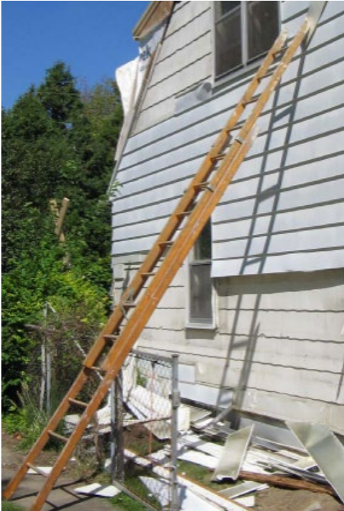
Photo from MIFACE report 05MI163 . The ladder is does not have safety feet, was not secured, is leaning against a moveable gate and is not following the 4:1 Rule.
