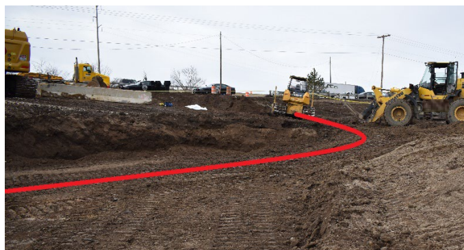
The red line shows the approximate path of the bulldozer through the worksite.
