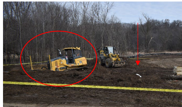
Location where the incident occurred. The bulldozer involved is circled. Location where victim was struck shown with an arrow.
