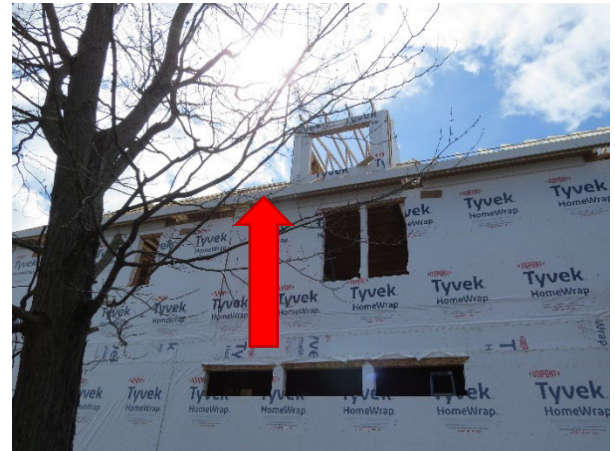
Ground view of the 3 rd floor and roof overhang of the new construction home. An arrow points to where the carpenter was standing prior to the fall.
