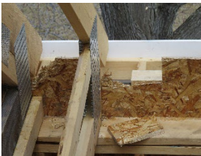
Location where the carpenter was standing prior to the fall.
