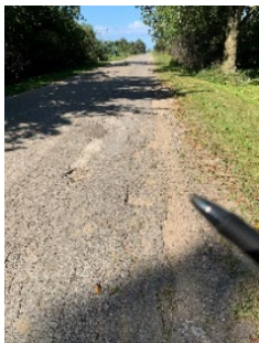
Roadway condition at incident site.
