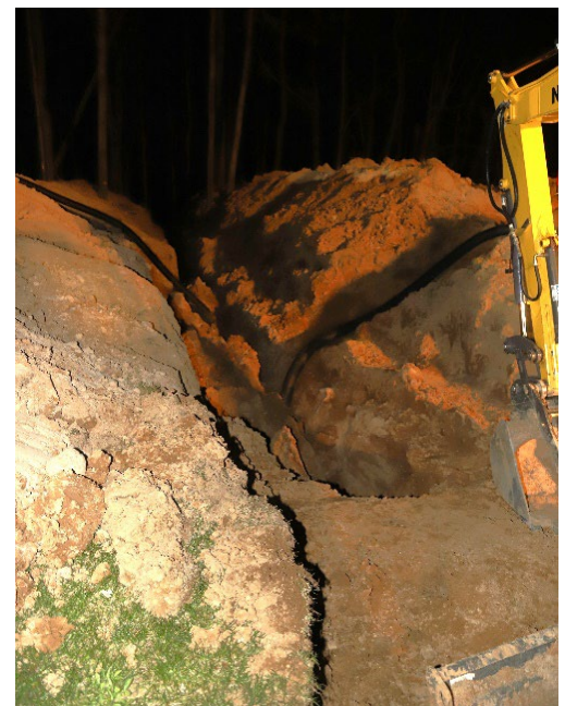
View of the collapsed trench prior to recovery efforts.
