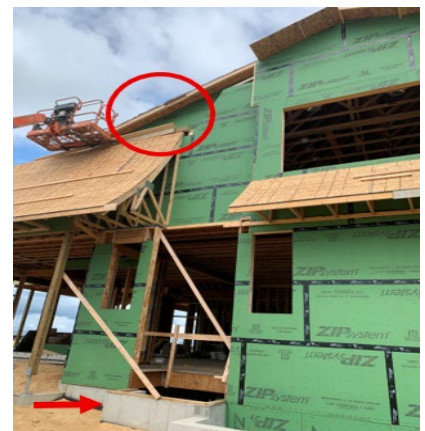
Red circle: area where the decedent and his coworker were working. Arrow: points to opening (hole) where the decedent struck his head. Source: MIOSHA
