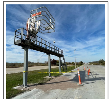
Ground view of the vendor platform with the gangway and platform in the raised position. Source: MIOSHA.
