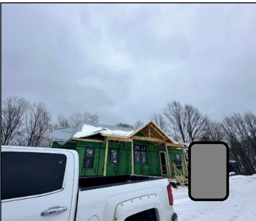
Front of house before tarp removal began. The tarp had to be cut at roof edge where scrap 2x4 was attached and holding it. The grey block excludes employees. Photo source: police photos.
