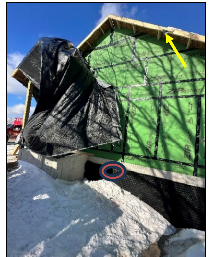
The tarp involved and victim's impact location (red circle) located on the right side of the house when facing the front. The yellow arrow indicates 2x4 sections used to attach and hold tarp on. Photo source: police photos.
