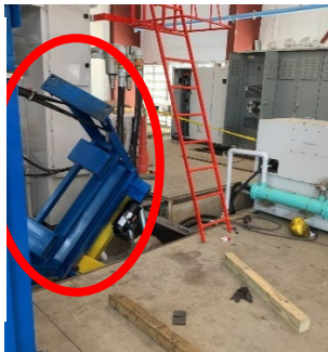
The fallen motor assembly (circled in red) and the wooden shipping blocks.
