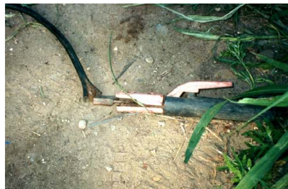
Figure 5. Un-insulated splice on bare ground
