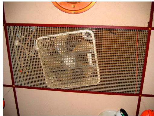
Figure 3. Fan laying on ceiling panel in bar area
