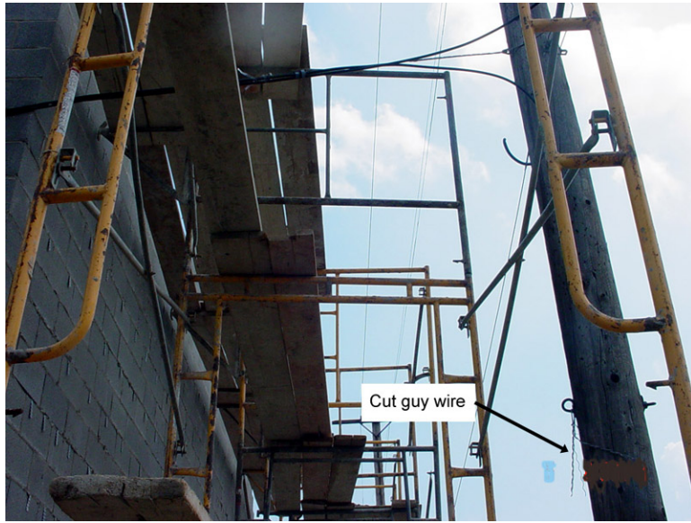
Figure 3. Photo showing cut guy wire
