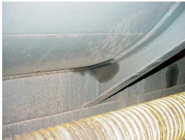
Figure 4. Leak location at base of tanker Compartment #3
