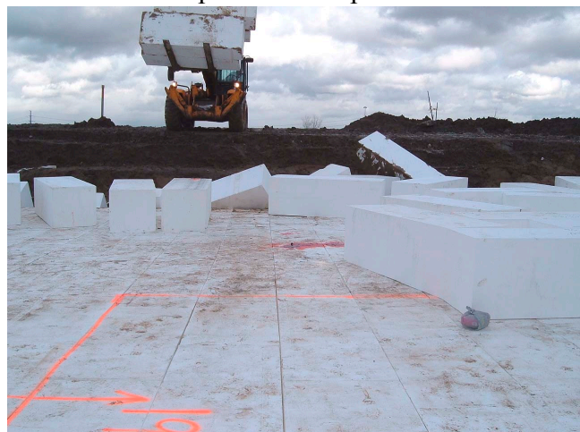
Figure 3. Incident site looking North
