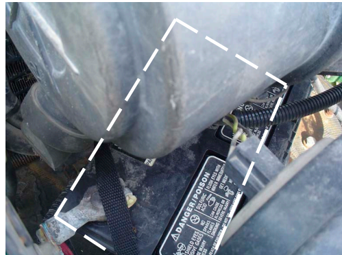
Figure 2. Sideways movement of battery
