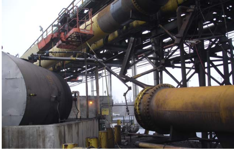
Figure 1. Incident Scene. 54-inch pipeline blown apart, area where patch repair occurred, and man lift used to elevate workers to pipeline repair area
