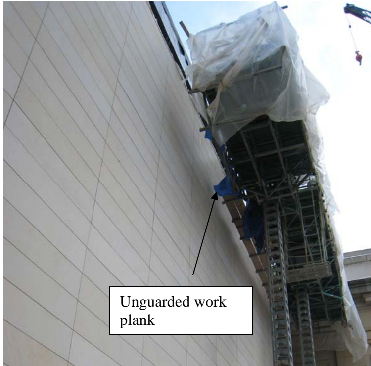
Figure 1. Unguarded north work plank on raised Hydro Mobile 2 scaffold
