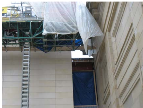
Figure 4. South working plank not guarded
