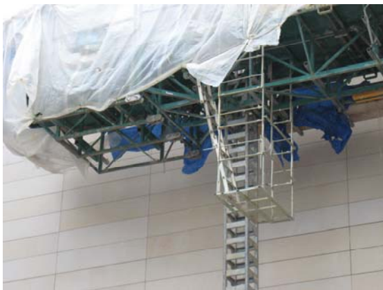
Figure 3. North working plank not fully planked nor guarded
