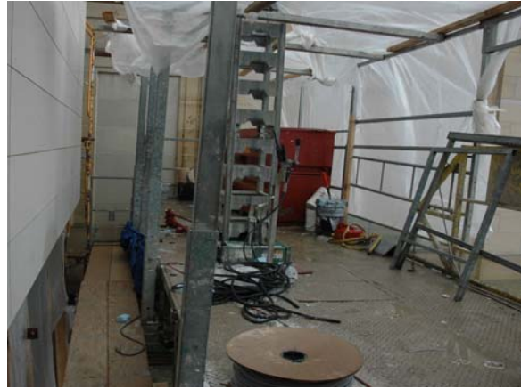
Figure 6. Guardrail installed on south end of working plank after incident
