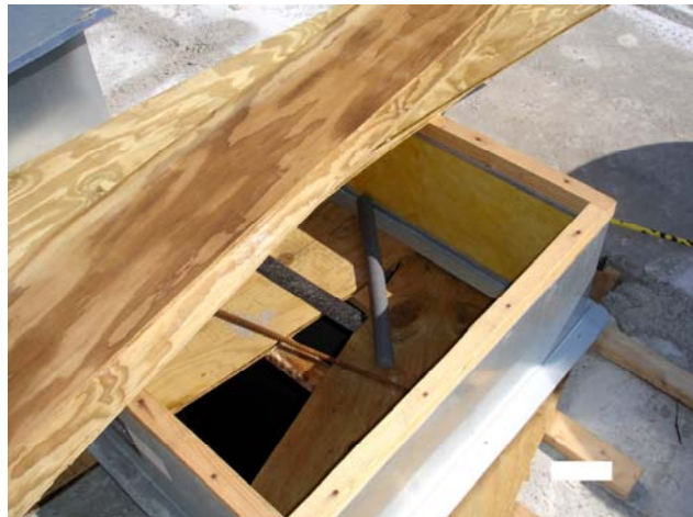
Figure 4. Chase A exhaust fan hole with 2x4 lumber and plywood boards as cover
