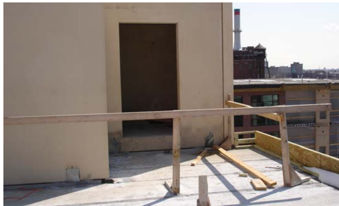
Figure 2. Guardrails at stairwell opening
