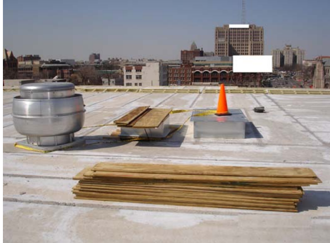
Figure 7. Make-up air roof curb with orange pylon, exhaust fan roof curb with plywood, looking north on roof
