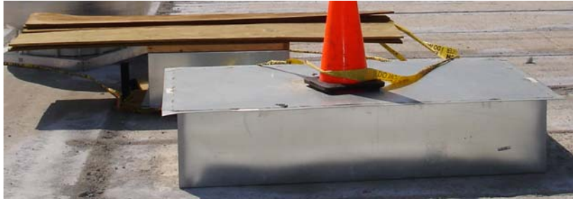
Figure 5. Close-up view of make-up air roof curb with cone, exhaust fan roof curb with plywood, looking west
