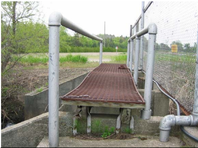
Figure 4. Water level control structure's wood and expanded metal walkway, handrails, and fence, looking south
