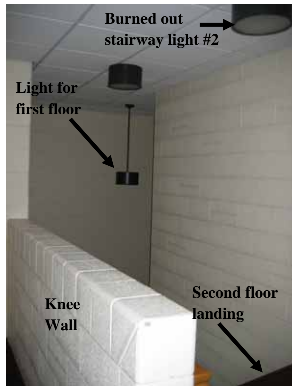
Figure 3. Standing on second floor landing, knee wall and burned out light
