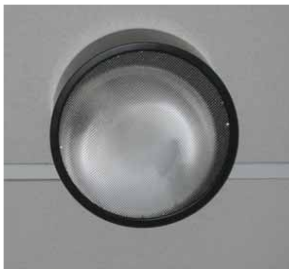
Figure 4. Burned out light in incident
