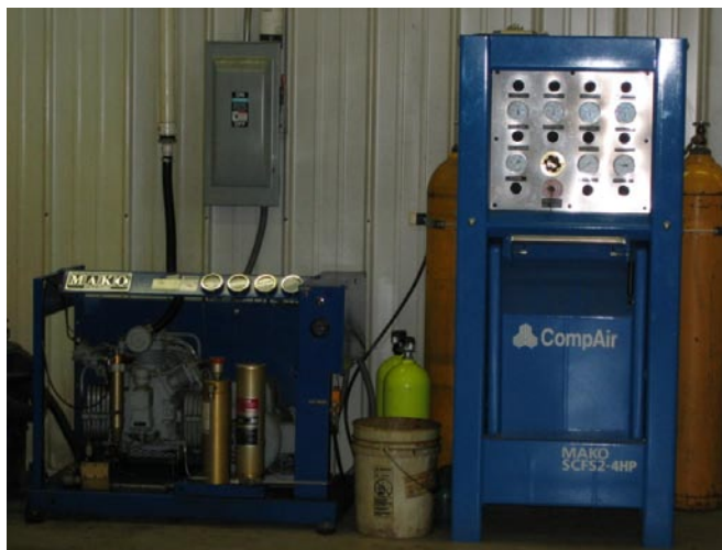
Figure 2. Air compressor and tanks
