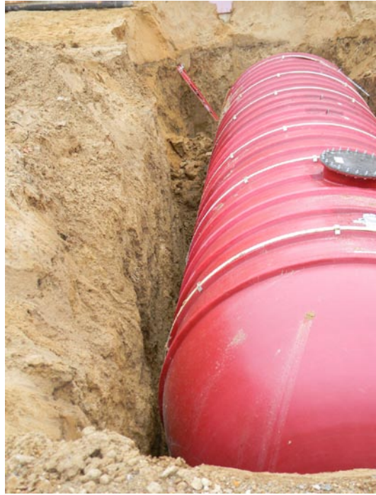
Figure 5. Collapsed soil in northwest corner causing tank to pivot to the east trench wall
