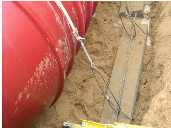
Figure 3. Concrete deadman anchor, steel rod and tie down straps on southeast end of water tank.
