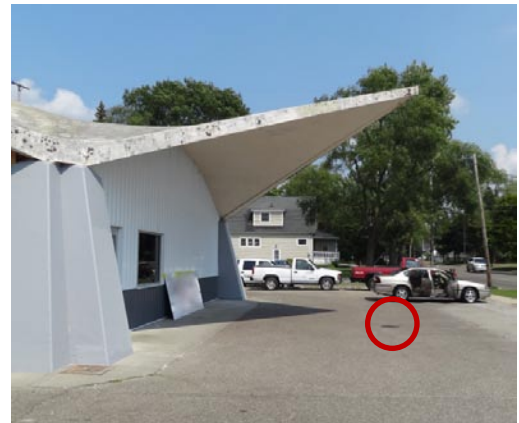
Figure 3. Example of building construction. Circle indicates drain location under tip of overhang
