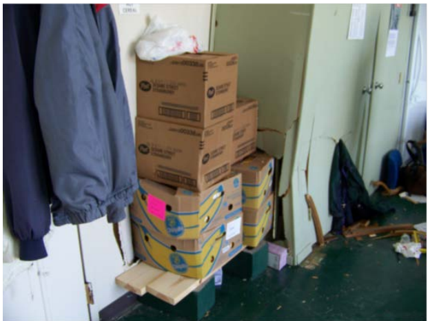
Figure 5. Damage to the west wall by the force of the table being pushed by the SUV
