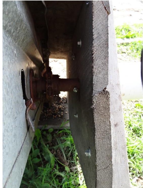
Figure 4: Unprotected PTO-elevator connection point with new PTO shaft shielding
