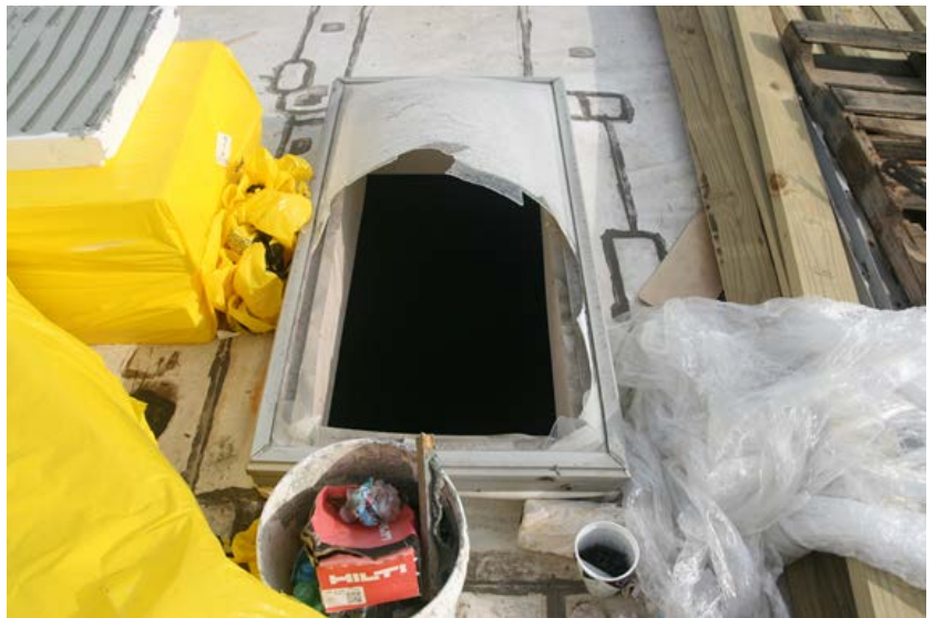
Photo 6. Skylight involved in incident
