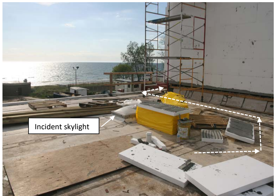
Photo 5. Incident area. Dotted lines show most likely path of decedent when he carried the prepared foam board to the owner working in the boom lift
