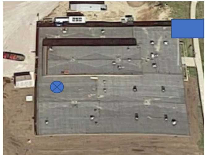
Photo 2. Water treatment plant building roof. Blue circle with X was approximate location of incident skylight. Picture courtesy of Google maps.
