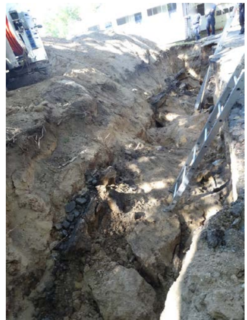
Photo 1. Overview of incident scene near driveway trench wall collapse, looking north.
