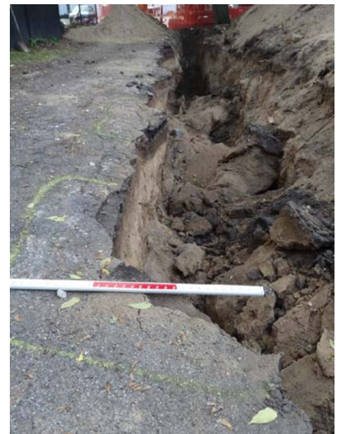
Photo 3. Area of trench wall collapse, looking south.
